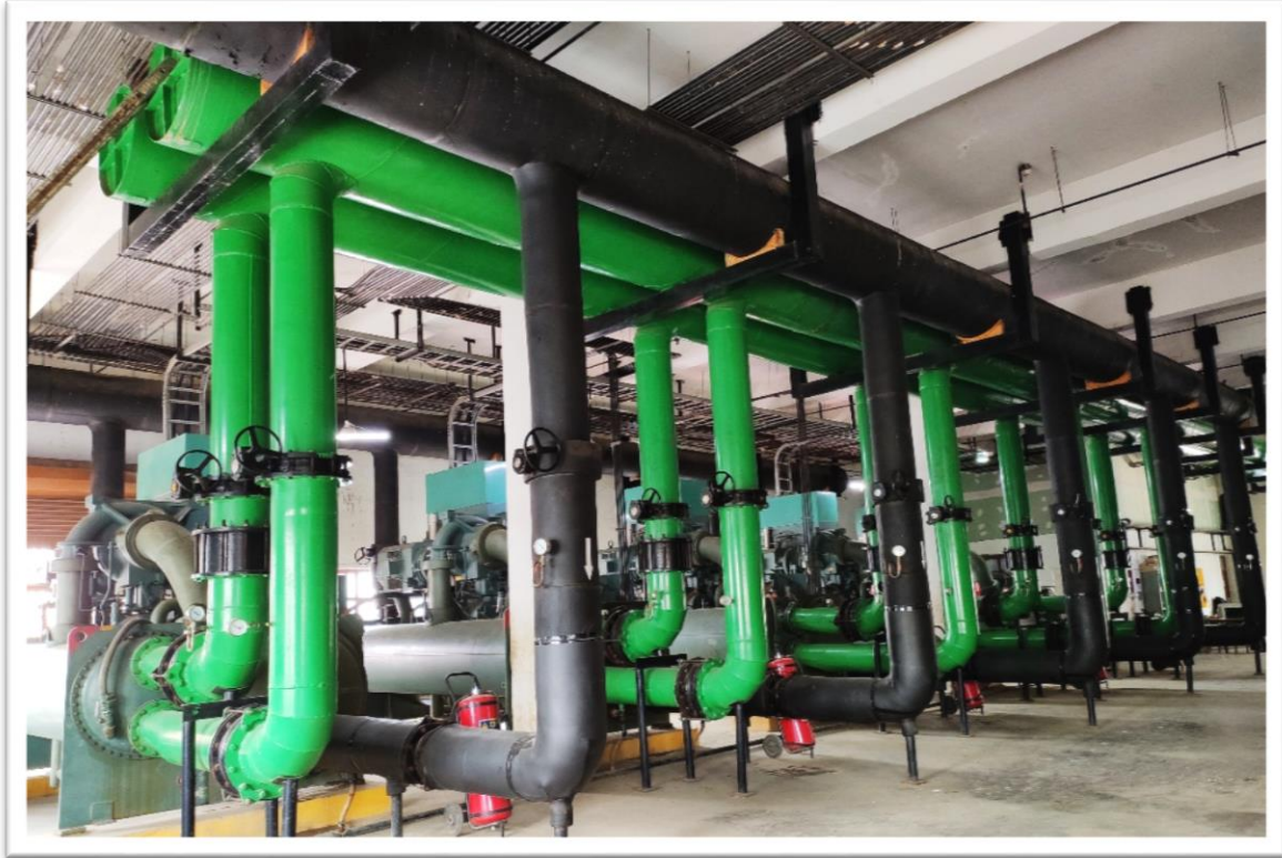
HVAC Plant Room
